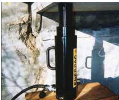
◀ The portable lock nut cylinder RACL-1506 used for extended load supports during epoxy injection for bridge reinforcement.
